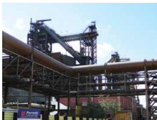
Fig. 4 – Gas coke pipe
